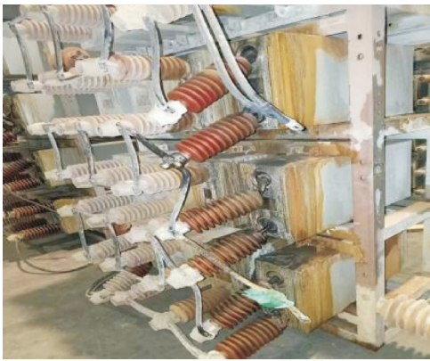
图8 重击穿后损坏的电容器组 Fig. 8 Damaged capacitor bank after restriking
