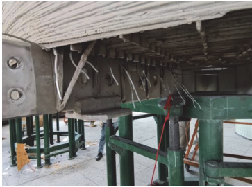
图 3 剥开后的电抗器出线接头 Fig. 3 The exposed reactor outlet terminal after being stripped
