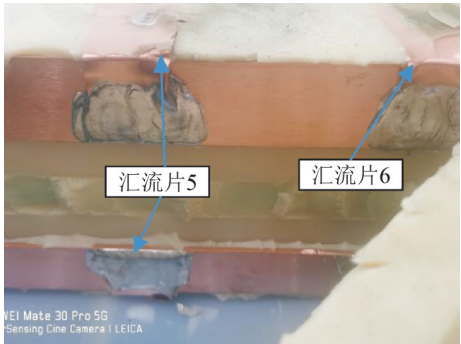
图10 2号试品的汇流排状况 Fig. 10 Busbar condition of No. 2# capacitor
