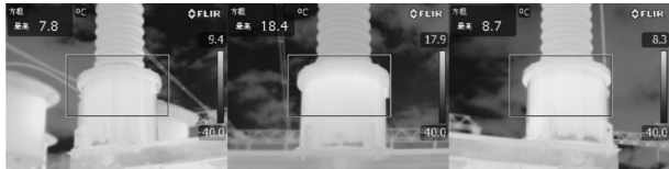
图 11 35 kV 电压互感器红外测温 Fig. 11 Infrared temperature measurement of 35 kV voltage transformer
