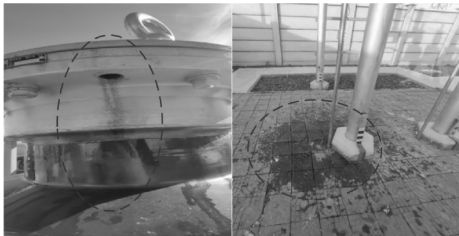
图2 电压互感器顶部漏油 Fig. 2 Oil leakage on top of voltage transformer
